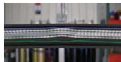
A damaged conduit can cause friction between the wire and the conduit and lead to friction and debris.
